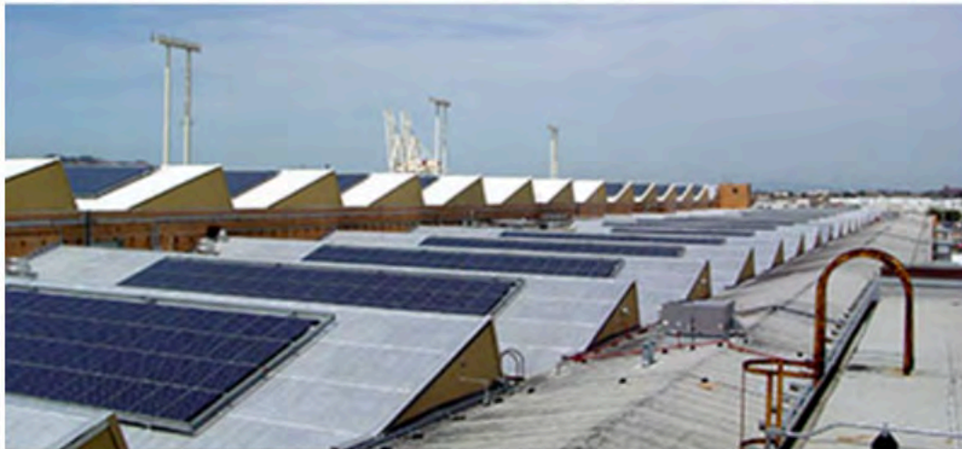
Figure 23. Solar collectors installed in a compatible manner on low sloping sawtooth monitors. Top Photo: Neil Mishalov, Berkeley, CA.
